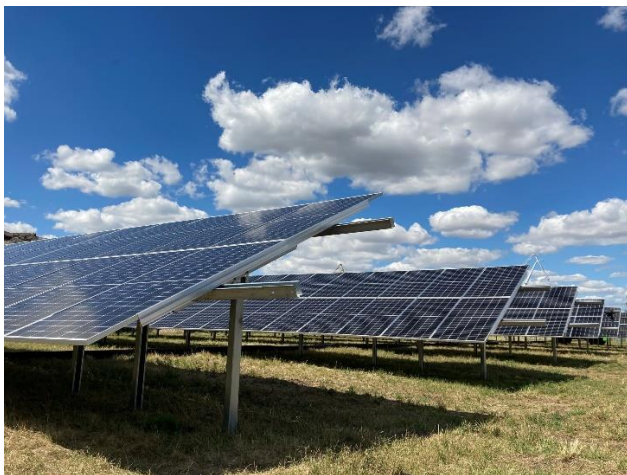
Photovoltaic solar panels on the ground
