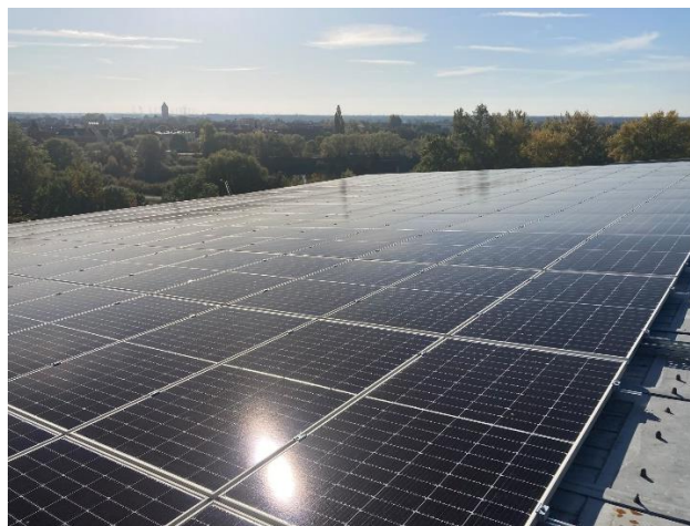
Photovoltaic solar panels on the roof of the plant
